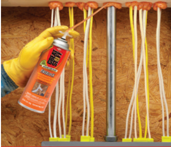
Electrical penetrations through floors
